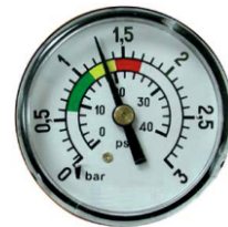
1,3 kg/cm 2 - 18,5 PSI: Proceed with Backwash operation
